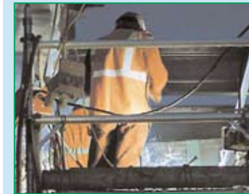
Mobile scaffold towers must be erected correctly
