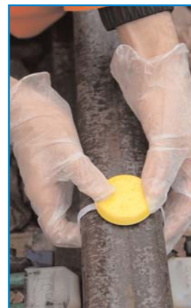
Detonator protection isn't placed at junctions
